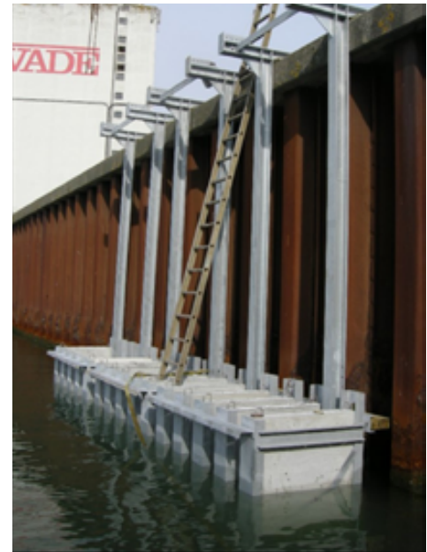
Large-sized concrete specimens (0.2 m × 1 m × 2 m) from marine exposure site at Rødbyhavn, Denmark. Image courtesy of Springer.
