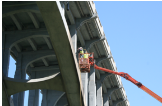
Inspection of a concrete structure to identify corrosion conditions. Image courtesy of C. Andrade.
