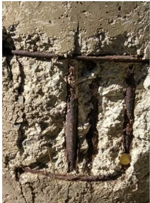
Advanced corrosion of steel in concrete. Image courtesy of S. Kessler.
