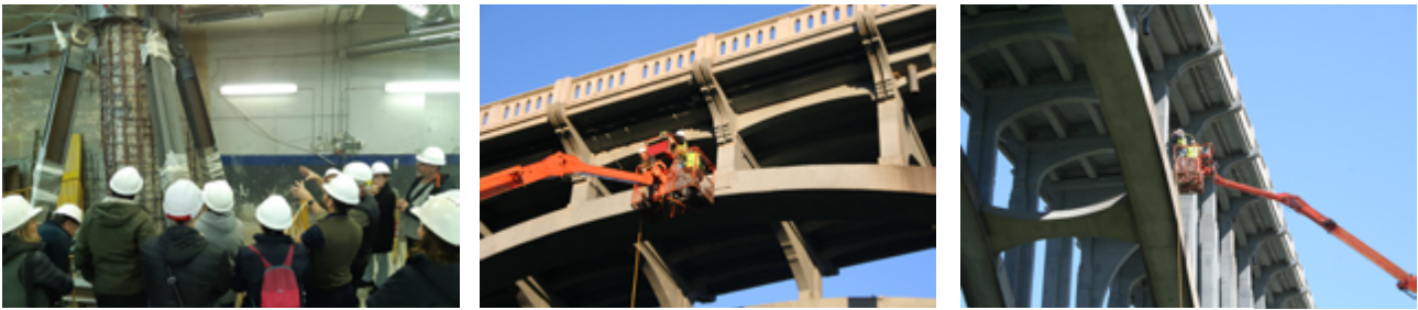
Observing a column with corrosion ©Carmen Andrade
