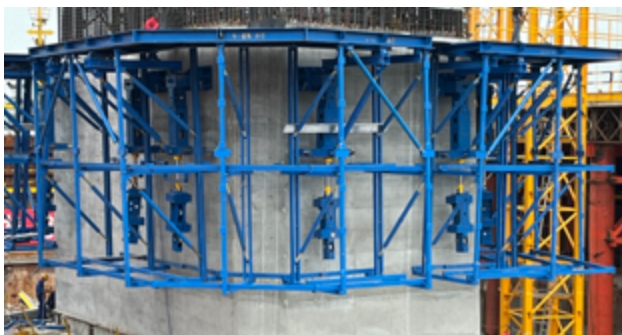
On-site application of concrete containing MgO and CaO-based expansive agent ©Jiangsu Sobute New Materials Co., Ltd., TC 284-CEC
