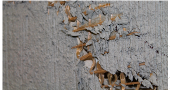
Failure of FRCM-strengthened masonry wall accompanied by fibers slippage. Image courtesy of the University of Salento.
