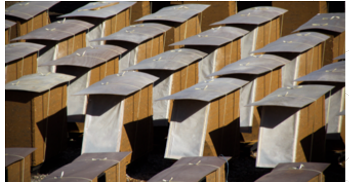
On site prefabricated rammed earth walls before being assembled, Lyon, France. Image courtesy of Clément Vergely Architectes.
