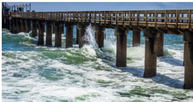
Concrete piers of the Swakopmund jetty in Namibia. Picture courtesy of Grant Durr.
