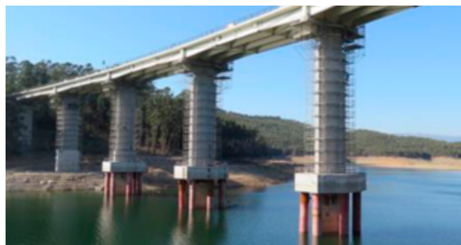
Bridge support pillars repaired after being damaged by alkali-aggreated reaction. Image courtesy of L. Oliveira Santos.
