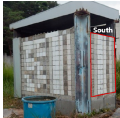
Experimental campaign to measure the durability of concrete panels coated with different finishing materials. Image courtesy of K. Imamoto.
