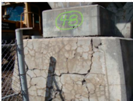
A concrete pylon damaged by alkali-aggregate reaction. Image courtesy of L. Sanchez.
