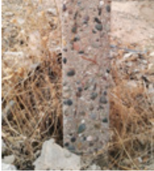
Spalling of concrete column in salty soil. Courtesy of Mu Song.
