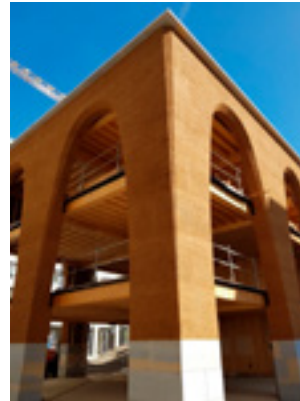
An office building under construction in Lyon, France: unstabilised rammed earth load-bearing 3 storeys; architects: Clément Vergely; Masons: Nicolas Meunier; Structural engineers: Batiserf. Courtesy of Batiserf.
