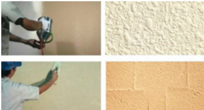
Coating the walls of buildings. Courtesy of Japan Building Coating Materials Association.
