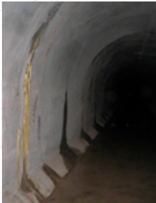
Leakage from cracks in a concrete tunnel. Courtesy of F. Kanavaris.
