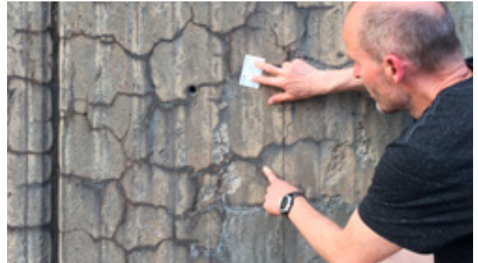
Measuring map-cracking of AAR in field. Courtesy of B. J. Wigum.
