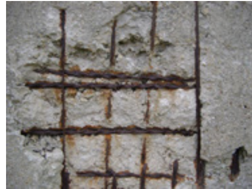
Corroded rebars. Courtesy of freeimageslive.co.uk.
