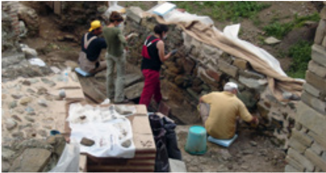
Applying lime based mortars on site Galerius Palace Thessaloniki 4th century BC. Courtesy of M. Sarantidou, Architect.
