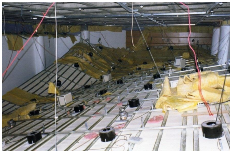
Figure 5: Ceiling collapse in educational building (source: [14]).
