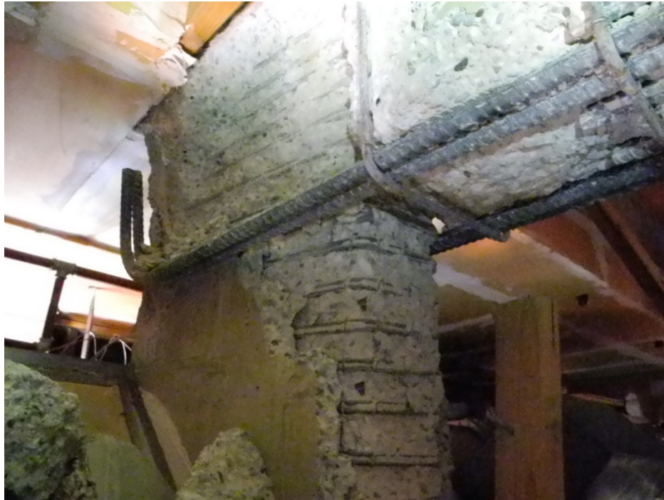
Figure 2. Failure of Transfer Beam, Copthorne Hotel, Christchurch (Photograph courtesy Peter McBean, Wallbridge and Gilbert).
