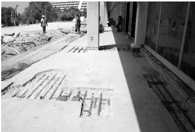
Photo 3: Slab above the service corridor: reinforcement exposed after removing the damaged concrete.
