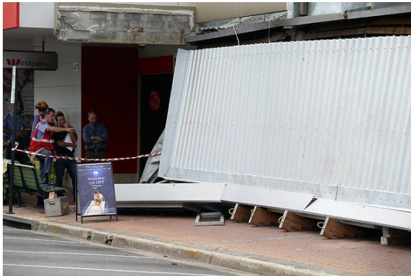
(a) Structure that swung down.
