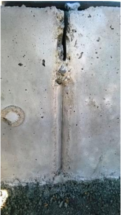
Fine crack in saw cut joint
