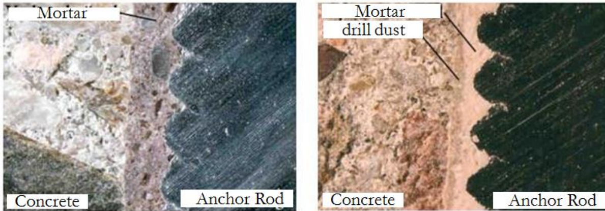
Figure 9. Cut sections of installed bonded anchors. The photo on the right shows a layer of drill dust between the adhesive and concrete (Courtesy of IWB, University of Stuttgart).
