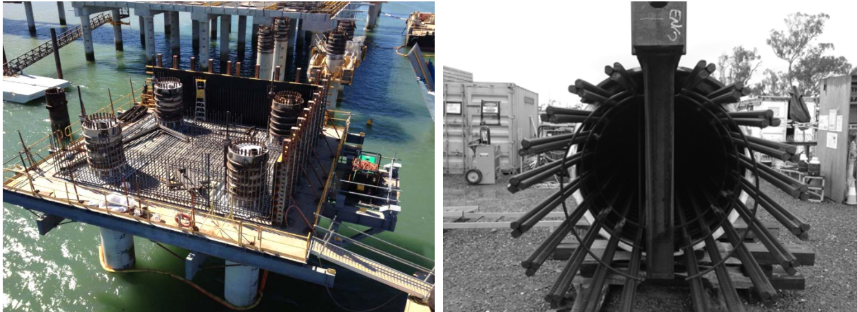
Figure 11. Left: Berthing Dolphin Construction. Right: Mooring Dolphin Pile Plug Temporary Works Assembly. @Arup
