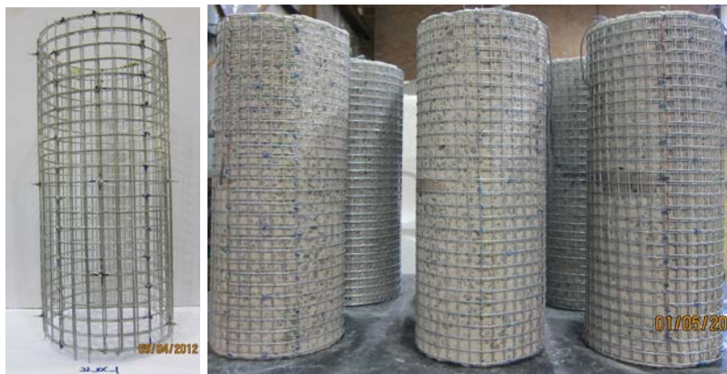
(a) Wire mesh cage (b) Wrapping mesh onto the precast core Figure 1. Wire mesh reinforcement installation
