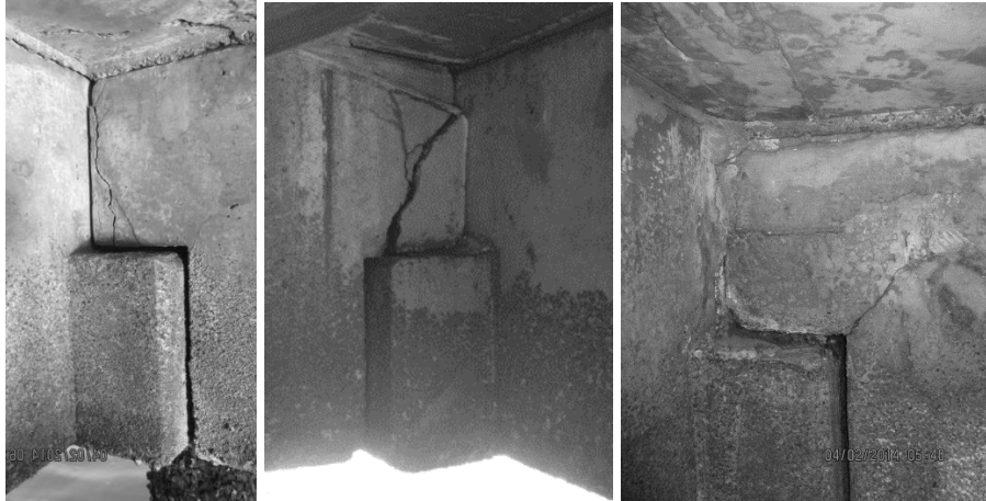
Figure 8. Jetty Finger Half Joint Cracking Examples. @Arup
