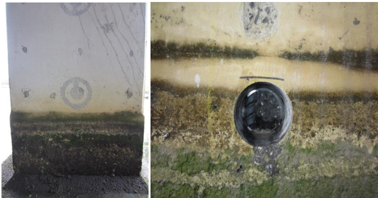
Figure 2. (L) Coating removed for measurement, some corrosion stain visible at construction joint. (R) Reinforcing steel at tidal/splash zone with no sign of corrosion.
