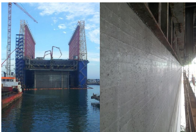
Figure 1. Caissons construction method. Right) Kugira floating dock, and left) detail of the bottom part of the sliding formwork.
