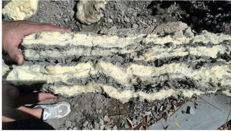
Figure 2. Sandwich structure of grouting material foam layer and graded broken stone layer.
