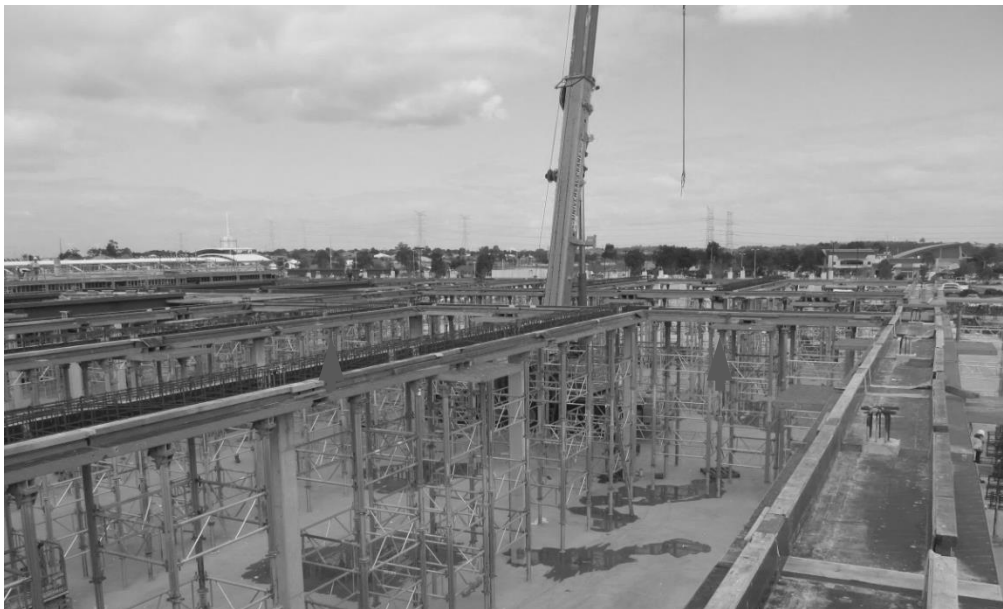
Figure 11. Linear formwork arrangement and use of P/T slab as high-capacity working platform
