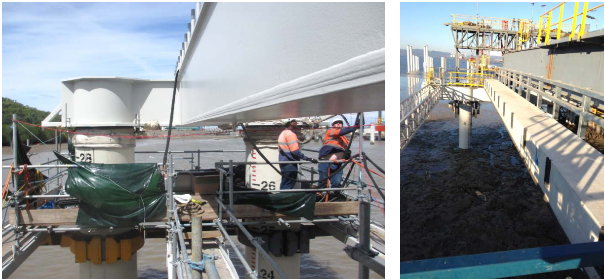
Figure 3. QCLNG Trestle. Left: Headstock (Anchor Bent) During Welding to Pile. Right: One Deck Unit Installed. @Arup
