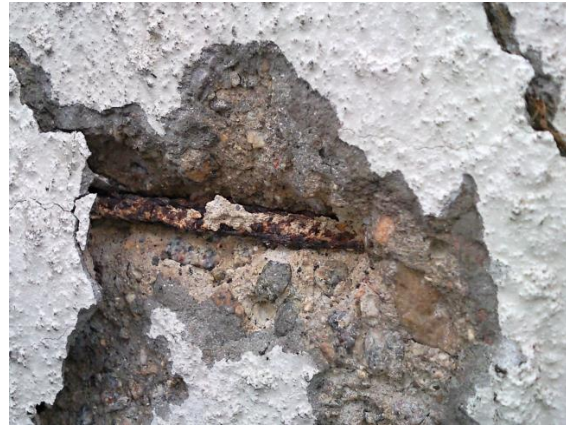
Figure 2. Detail of a corroded bar; surrounding concrete is damaged by expansion of corrosion products.
