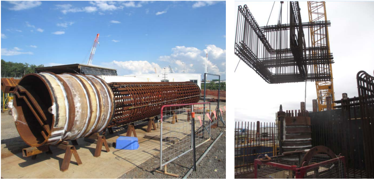
Figure 9. Left: Berthing Dolphin Pile Plug Prefabricated Assembly. Right: Modular Reinforcement Being Lifted into Pile Cap. @Arup
