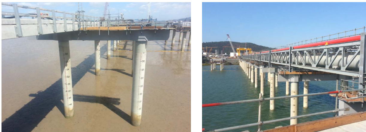
Figure 4. GLNG Trestle. Left: Typical Bent View without Pipe Rack Modules. Right: View after Pipe Rack Module Installation. @Arup
