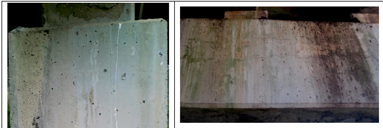
Figure 1- Mild cracking in column (left) and crosshead (right) of Bridge A
