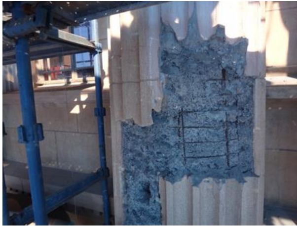
Figure 6 – Fluted column following removal of defective concrete with corroded reinforcement cage visible
