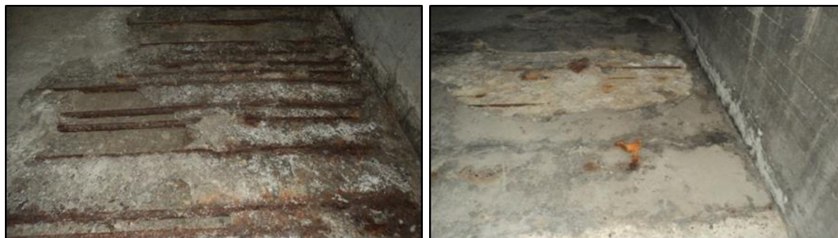
Figure 1: a) Inspected floor and ceiling of the ventilation tubes in the tunnel b) damage continuation in the previously repaired patches
