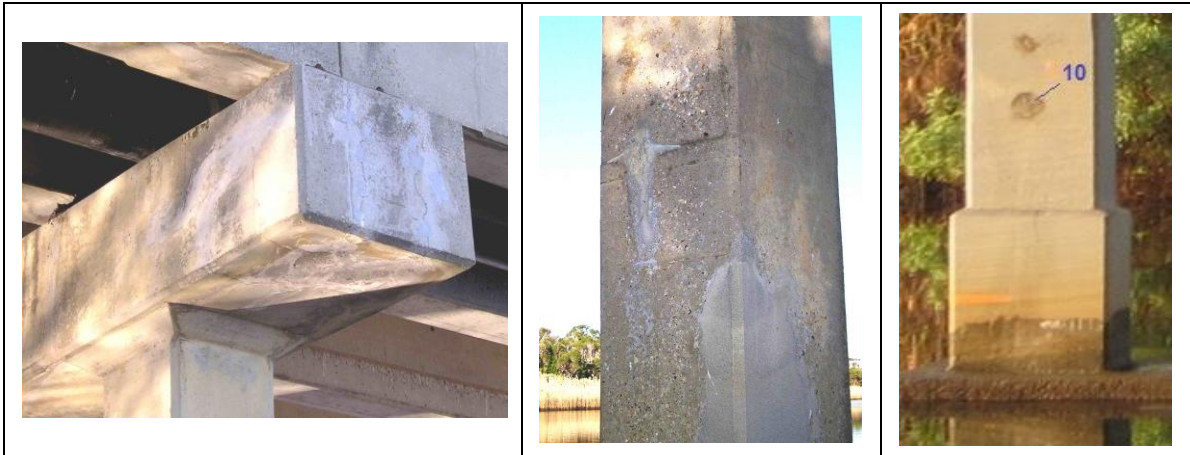
Figure 3- Views of repair in a crosshead and a column in Bridge C. Note jacket at the base of column applied later for scour protection
