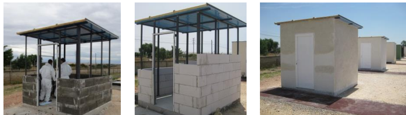
Figure 7. Testing cells being built with GREEN CAST blocks (left) and Ytong ones (center). Both testing cells finished (right).
