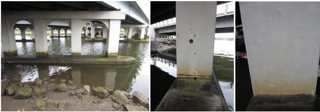
Figure 1. (L) Pier 2 Lynch's bridge (inbound), (C) Middle column of pier (P2C3) and location of cores. (R) Column P2C5- crazing, small spots of damage.
