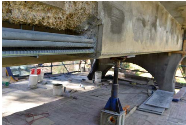
Figure 8 The existing & new reinforcement together with new concrete to half of an external beam
