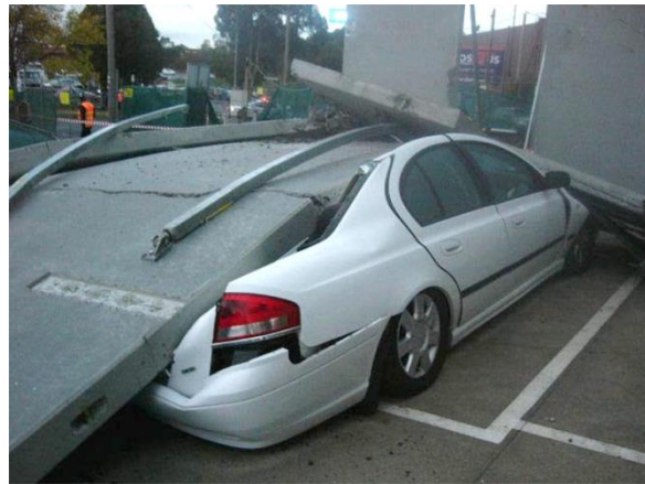
Figure 2: Precast panel failure during erection crushes cars (source: [8]).
