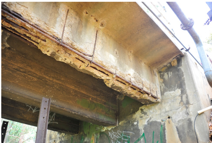
Figure 4 A view of the worst external beams 2011, which was the trial beam, repaired in 2013.
