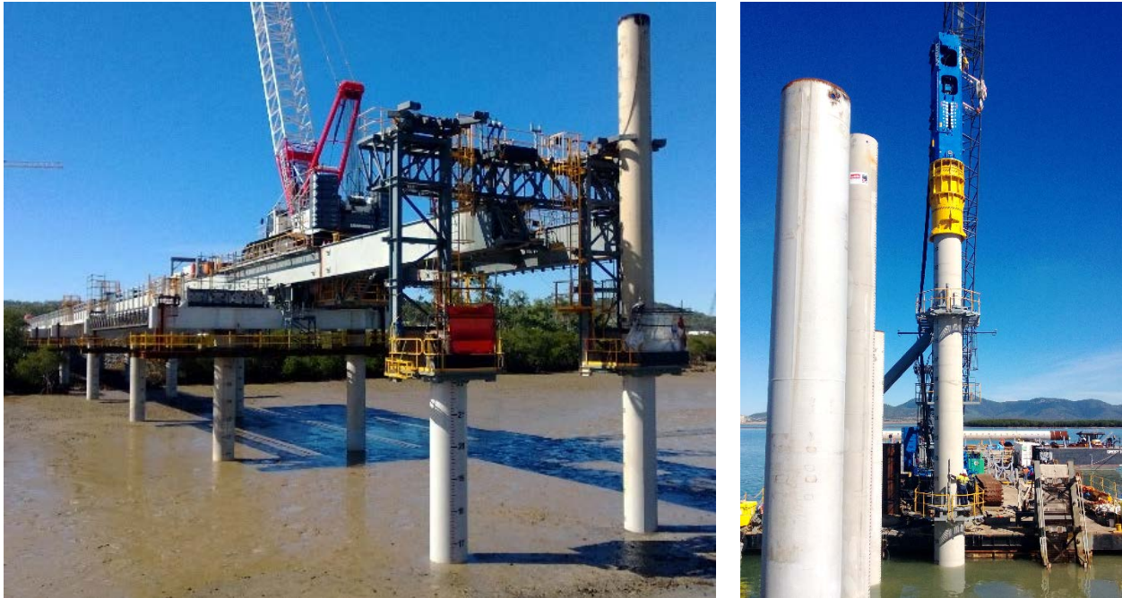
Figure 2. Example of LNG Jetty Piling (from Australia Pacific LNG). Left: Piling using Traveler. Right: Piling using Floating Barge. @Arup
