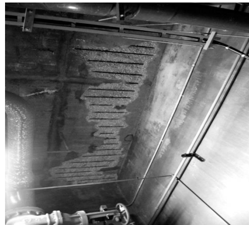
Photo 4 : Pump room slab: spalling of concrete and exposed reinforcement
