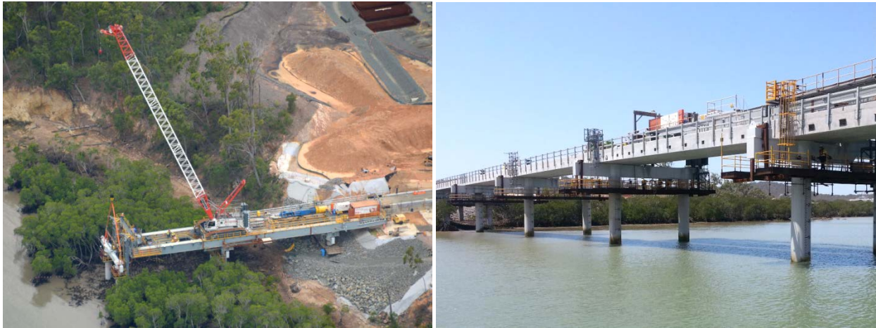
Figure 5. Australia Pacific LNG Trestle. Left: Traveler Trestle Construction. Right: Completed Trestle Roadway. @Arup
