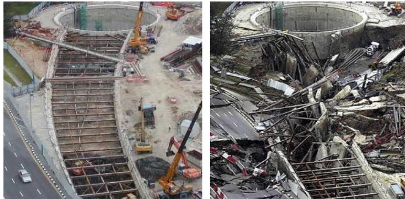
Figure 4. Singapore MRT Diaphragm wall collapse (Before and after), Singapore 2004 Photos reproduced from Chou (10)
