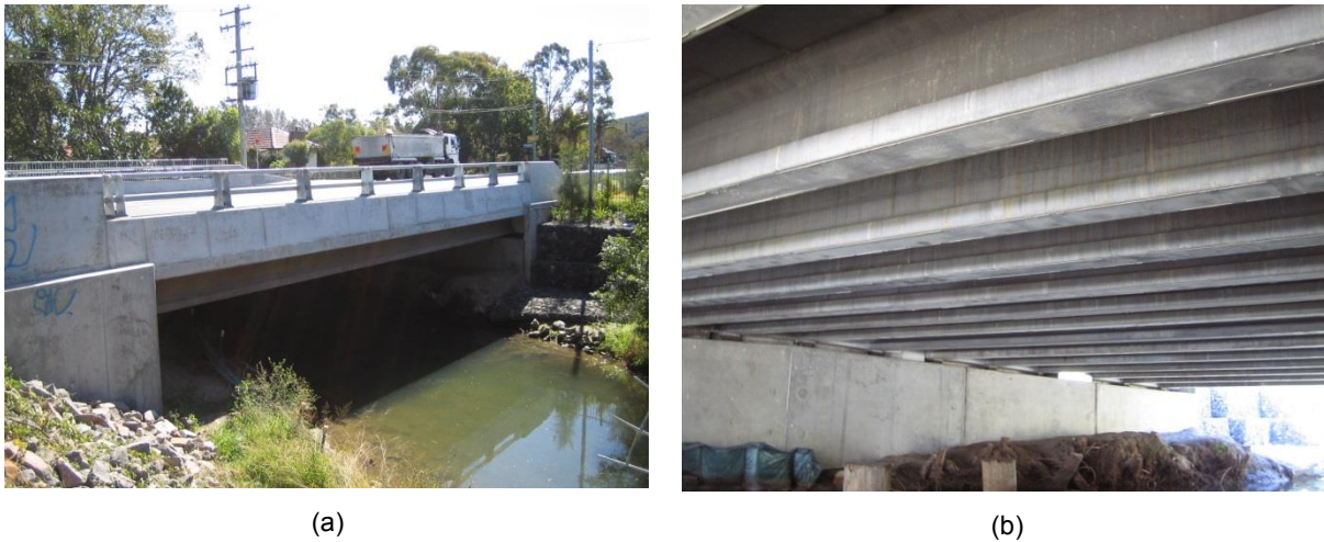
Figure 3. Shepherd's Gully Bridge, NSW, Australia constructed 2005: (a) 15 metre span 4 lane road traffic bridge (b) underside showing I-girders.
