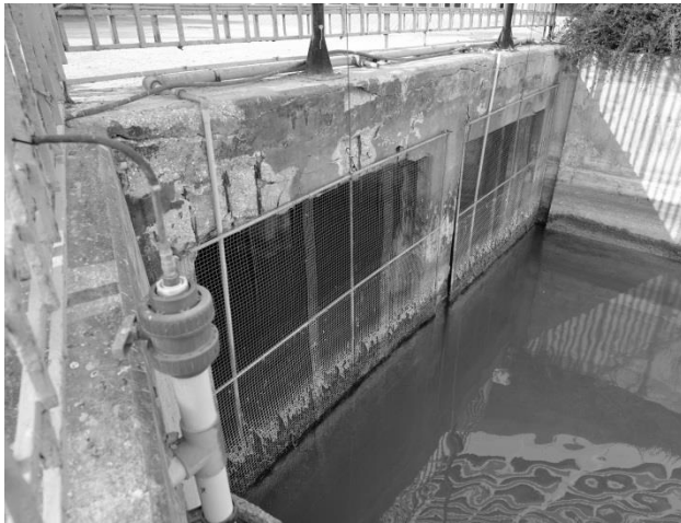
Photo 1- Sea water intake entrance beam: concrete spalling and reinforcement exposed.
