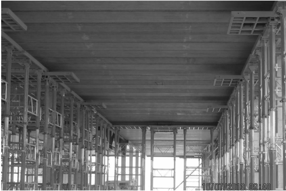
Figure 10. Linear formwork arrangement for supporting the planks and casting the P/T beam
