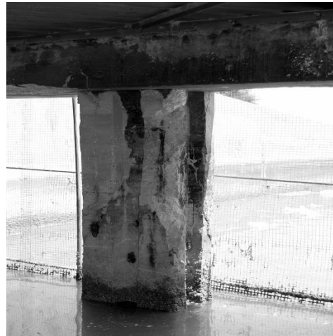
Photo 2 – Sea water intake column: Extensive damage to the concrete and exposed reinforcement
