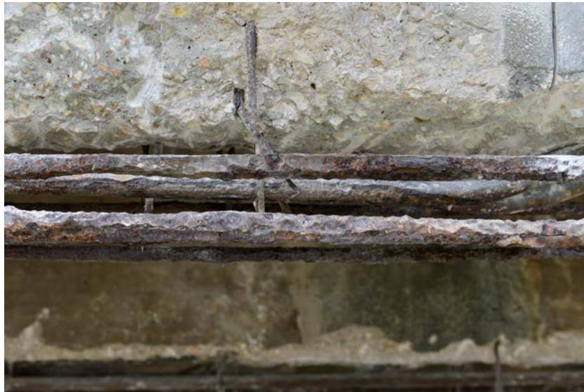
Figure 5 Corrosion of the original round reinforcement and the density of the uncracked concrete
