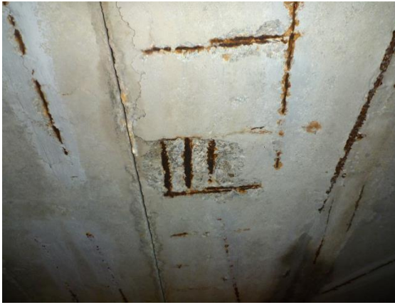
Figure 1. Corrosion of reinforcement in reinforced concrete structure.
