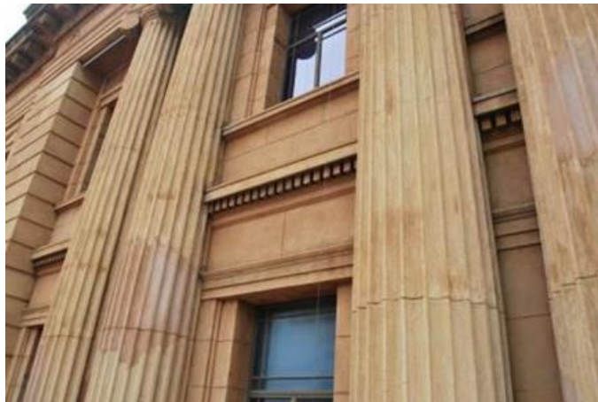
Figure 2. Precast columns undergoing carbonation North Façade.
