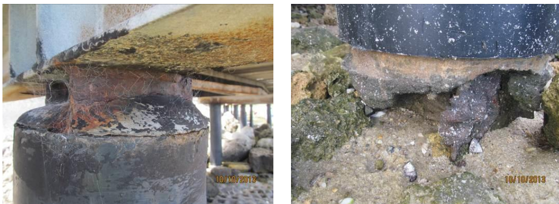
Figure 1. Left: Steel UC Connecting to Steel Framing. Right: Steel UC Below Concrete Encasing.
