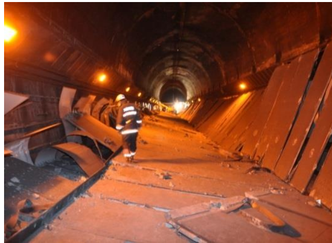
Figure 7: Partial collapse of concrete panels in Sasago Tunnel (source: [20]).
