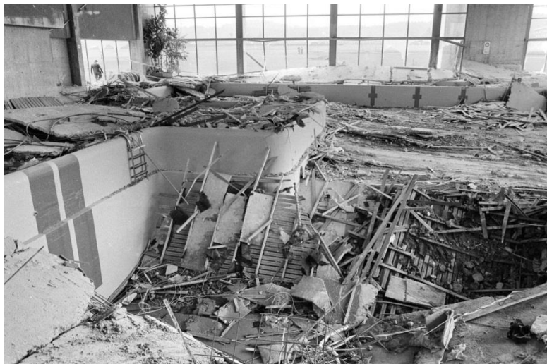
Figure 6: Collapse of heavy concrete ceiling in swimming pool facility (source: [17]).
