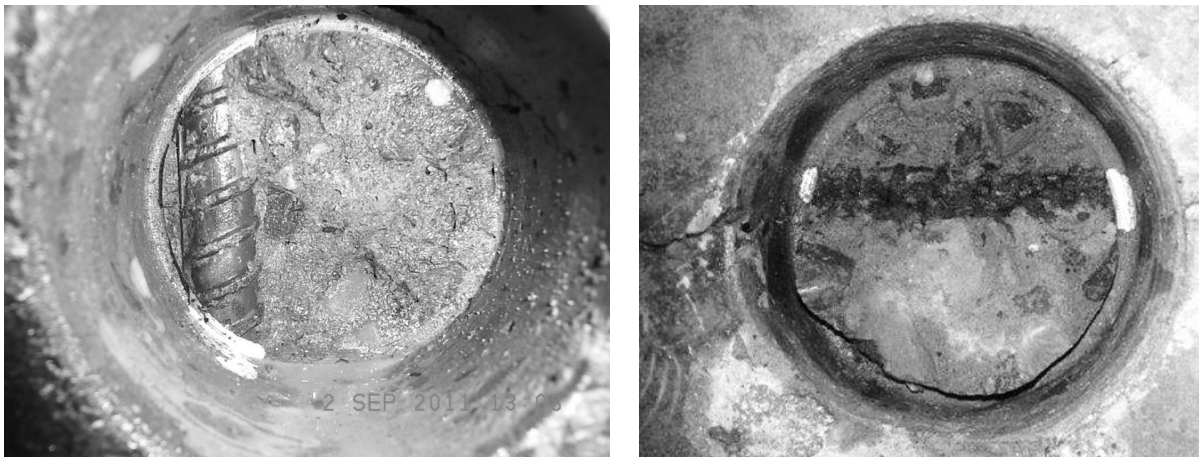
Figure 2 As part of the preliminary and subsequent investigations reinforcement was exposed for visual condition assessment. The bar in the left photo showed only slight superficial corrosion whereas the bar coincident with a crack in the right photo showed advanced corrosion.
