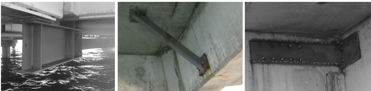
Figure 4. Examples of Installed Steelwork Supports. Left: Vertical and Torsional Support. Middle: Torsional Support. Right: Lateral Support. @Arup
