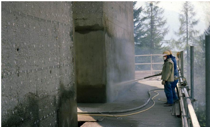
Figure 1: Shotcrete application for bridge column repair. Here shotcrete is embedding the anode grid of a cathodic protection (picture Kusterle)
